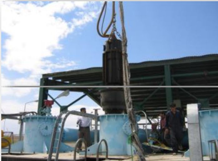
ARAS Dam Pumping Stations
