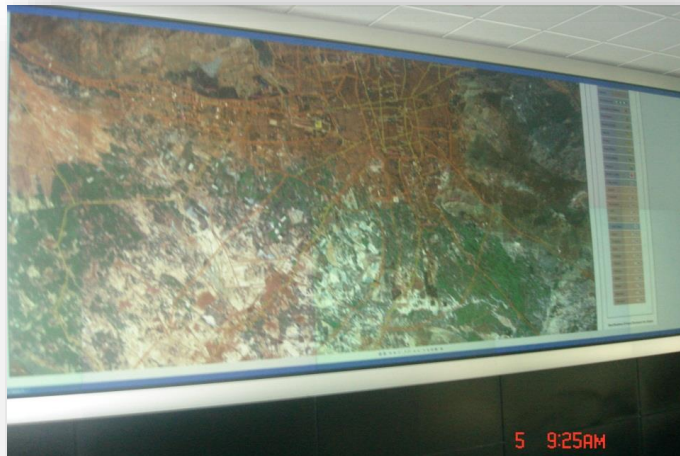
South TEHRAN Water Transfer Telemetry System
