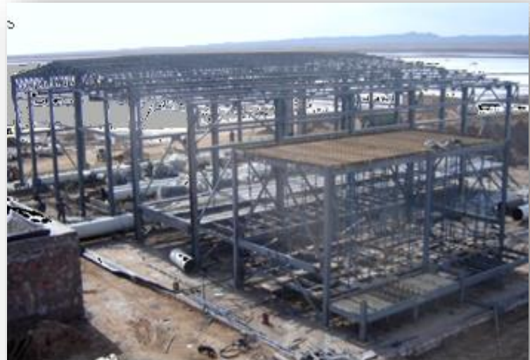
SHOORABEH Pumping Stations For POTAS Project
