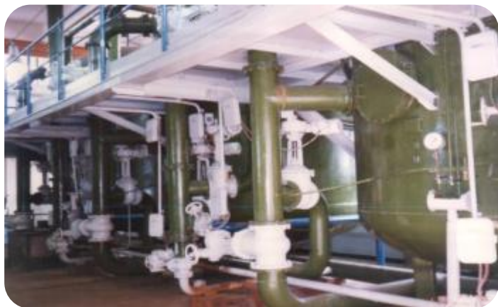
PARS Paper Factory Water Treatment Plant
