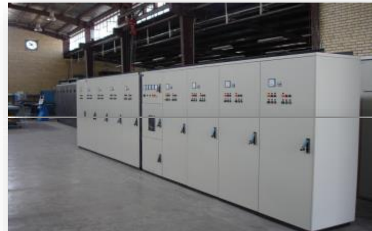
ALASHTAR Pumping Stations
